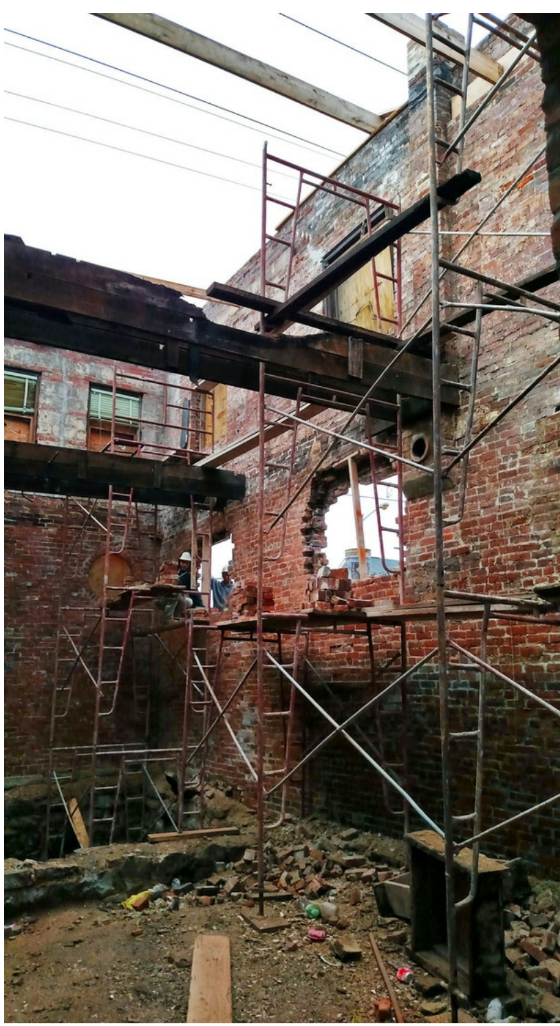
A look inside the building on Jo Johnston Ave. when the restoration work began.
