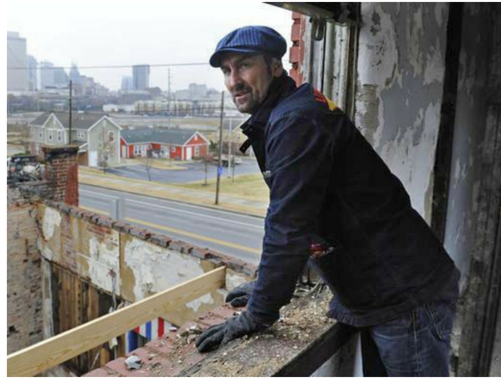
Mike Wolfe looks out the second story window of the building in 2014 before the renovation. (Photo: Shelby Mays/The Tennessean)
